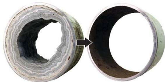
Figure 1 Pipe with scale deposits on the left and after scale removal on the right and [5]
