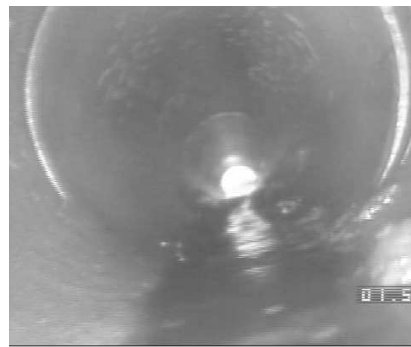
b. Joint misalignment and crack
