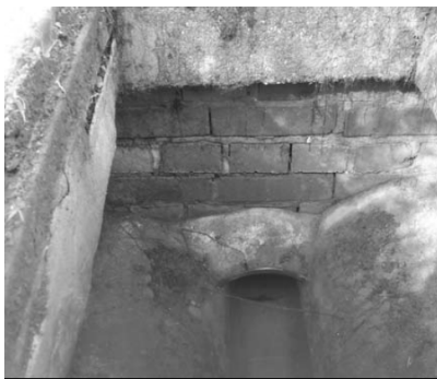
a. Damaged manhole joints
